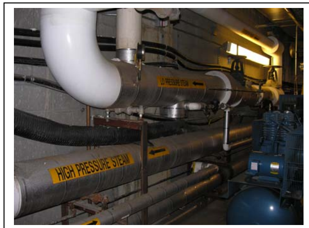
Figure 5: Steam Lines, communication lines, and electrical lines now run through the building and connect to underground tunnels on the other side of the foundation walls.
